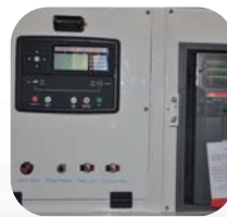
Control Panel & MCB
